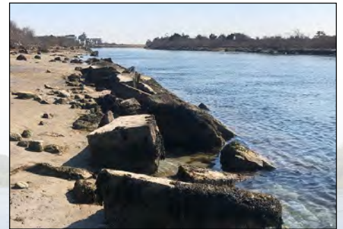
Previous failed attempts to control shoreline erosion at the Quonochontaug Breachway. New nature-based resilient designs are planned to more effectively address the effects of sea level rise and provide continued access to anglers.
